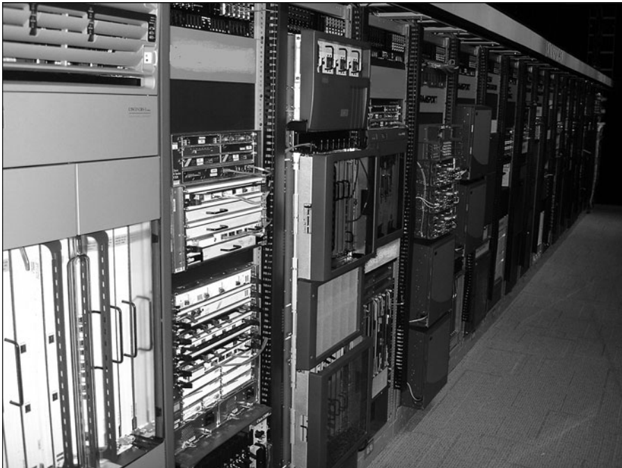
Figure 2-2 Rack-Mounted Network Equipment
